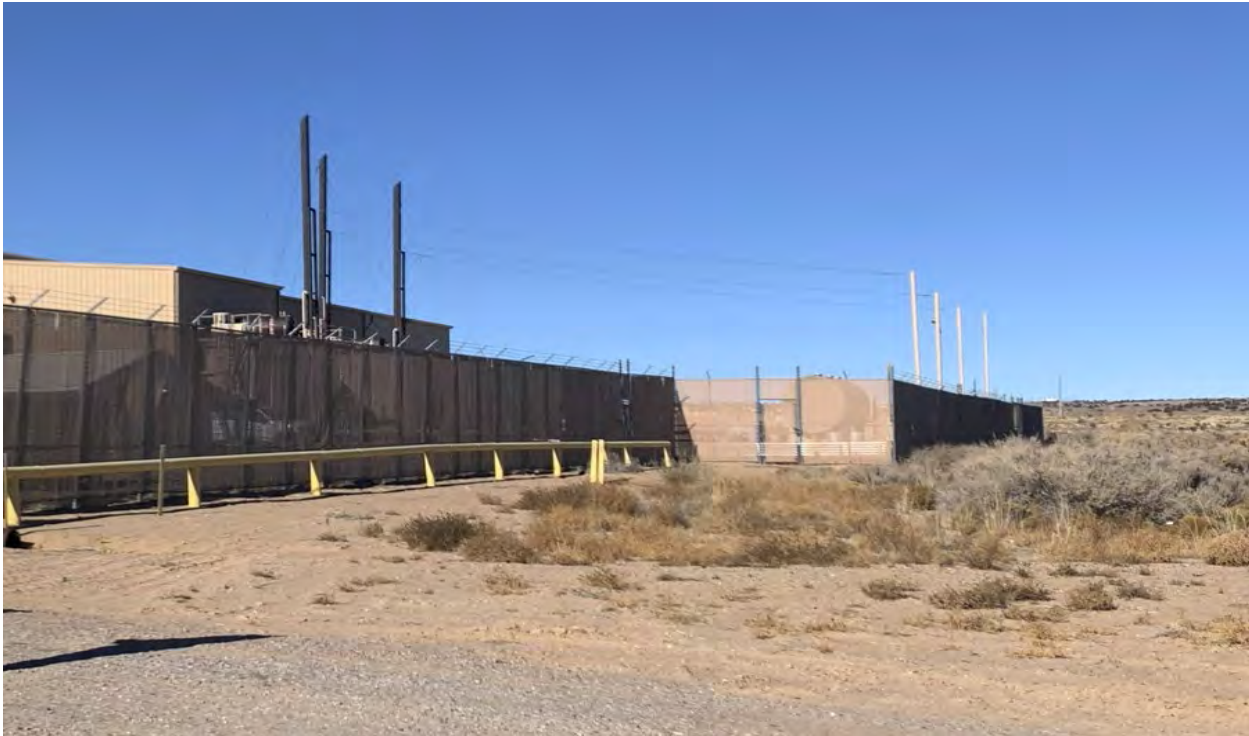
Figure 3. Espejo Compressor Station at Santa Fe Junction Site
